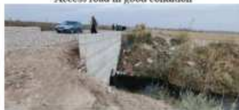
Side view of damaged bridge-1
