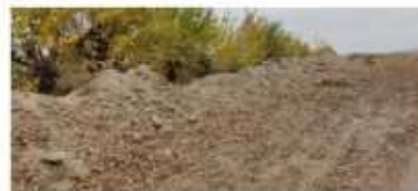
Loose earthen soil on the roadside
