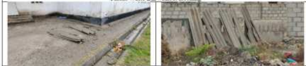
ACM left over at the school campus
