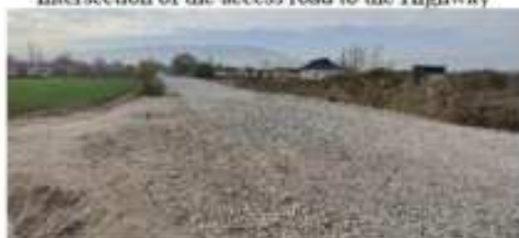
Damaged approach of Bridge-1
