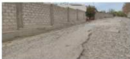
Damaged Paved Road
